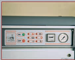
ELECTRIC PANEL Full compressor operation control.
